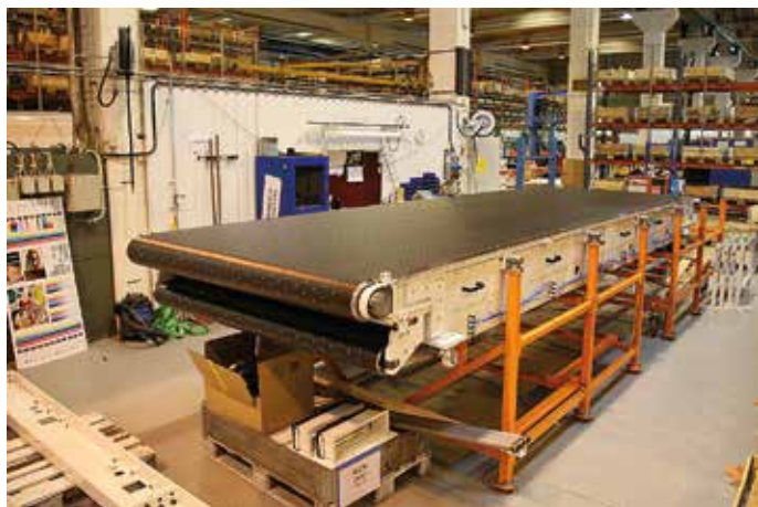
The feeder table is another part of the machine that is measured with Easy-Laser®. Here the aim is to check e.g. that the rolls are parallel and at right angles to the table.
